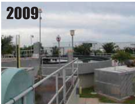
Titusville, FL , at city WWTP. Mounted near sewage digester, near air-conditioning unit, generator. RATING = CRN5
