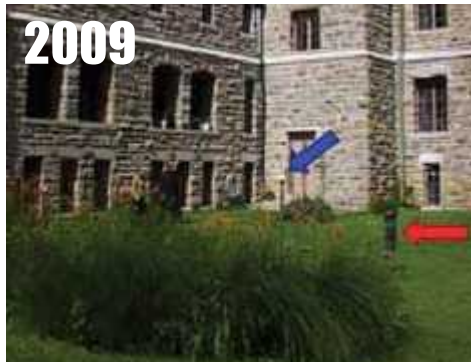
Atchison, KS , near corner of large stone buildings. RATING = CRN4
