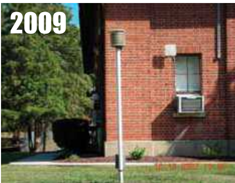
Salisbury, MD , nearby building, air-conditioning unit. RATING = CRN4
