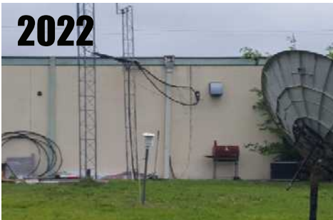
No change in location, but MMTS is now tilting due to lack of maintenance. RATING = CRN4
