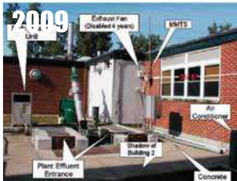
Urbana, OH , at city WWTP, mounted on brick wall, other multiple violations (see labels). RATING = CRN5
