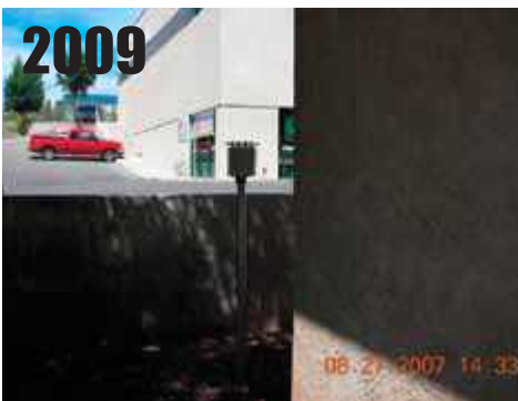
St. George, UT , between building and raised parking lot, car radiator level. RATING = CRN5
